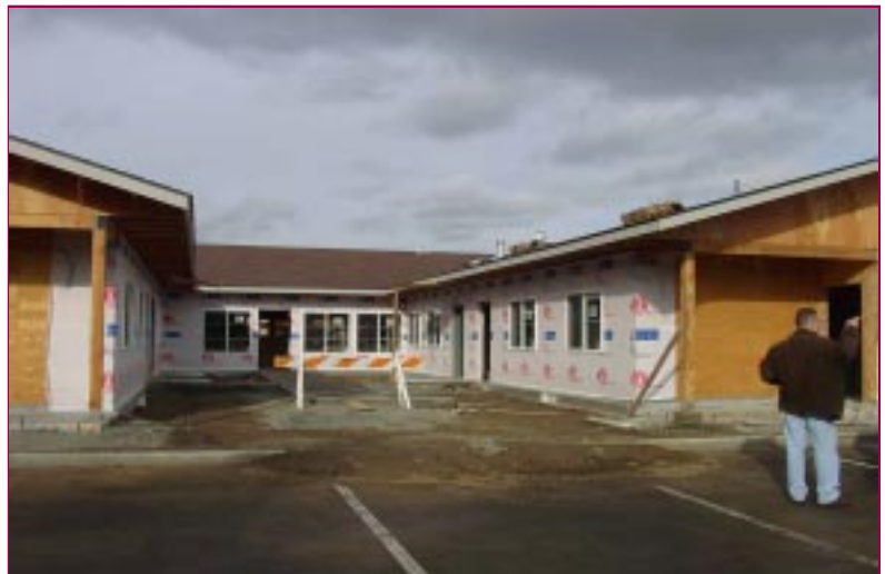
Construction Phase of the new building for the Riel House PPW Program
